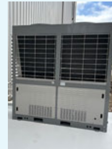
Figure 19: Parsons, KS Closed Loop Water System
